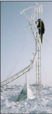
Collapsed tower, Flat Mountain, 1991.
