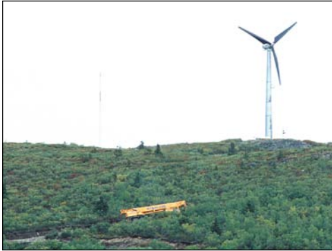
The crane used to erect the new tower on its way up the newly widened road towards the Bonus.
